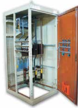
MV Capacitor Banks
